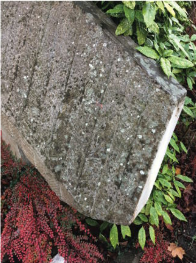
Figure 4.22 Lichen growth on a concrete surface.
