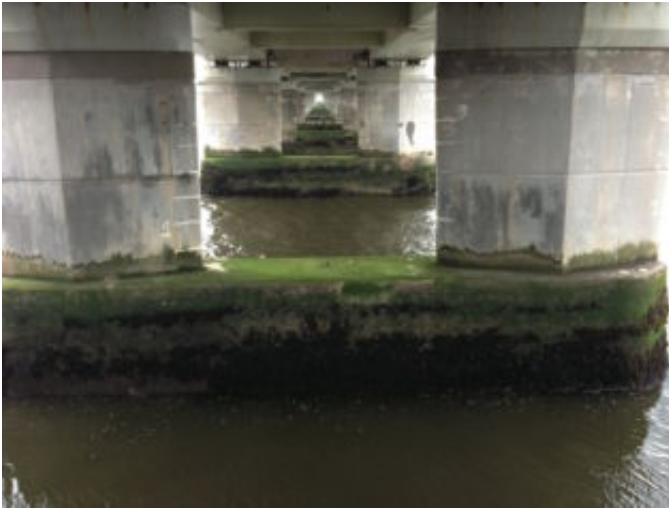
Figure 5.1 Algae in the form of an algal biofilm and seaweed at the waterline of a concrete bridge.
