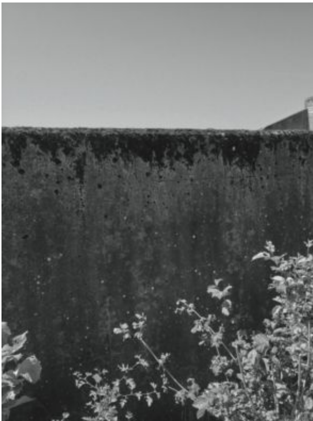
Figure 5.4 Moss on a concrete wall.
