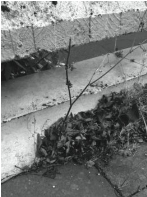
Figure 5.16 Plant growing in a joint in a concrete structure.
